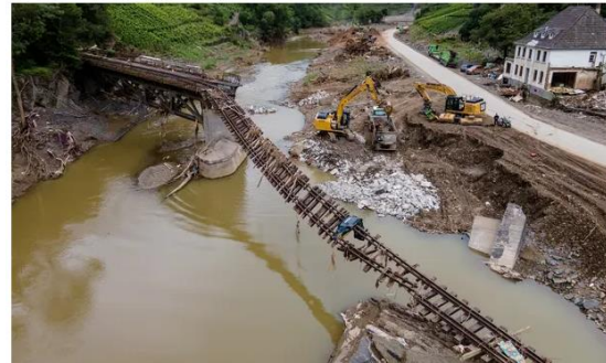
■ A damaged railway bridge five weeks after the flooding of the River Ahr in Rech in the Ahrweiler district of Germany on 19 August. Photograph: Friedemann Vogel/EPA
